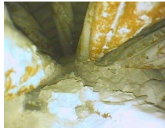
b) Inside view of a tendon in an externally post-tensioned bridge with large voids and corroded strands (TxDOT 2009)
